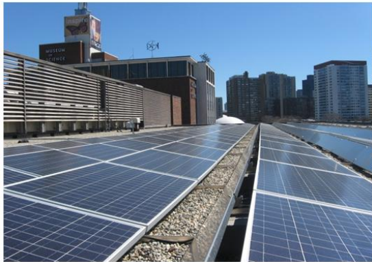
PV Alternative Energy Source
