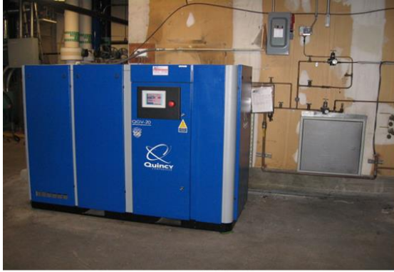
Compressed Air System
